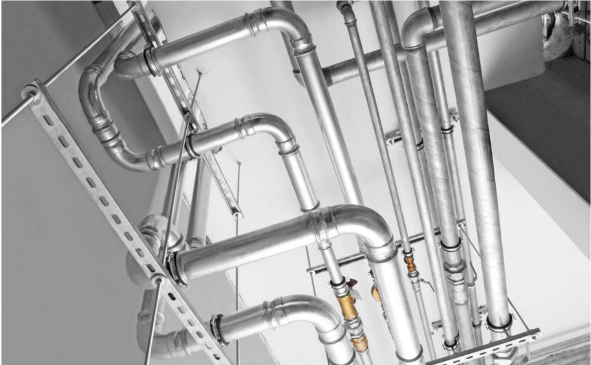
Exemplary KAN-therm Inox installation
